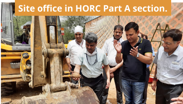
Ground Breaking Ceremony of Site office in HORC Part A section at Manesar held on 28.05.2022
